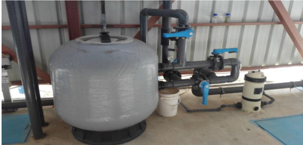
Figure 15: Disinfection unit at TRWWTP.
