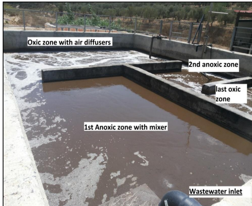
Figure 4: The AS Tank in AWWTP
