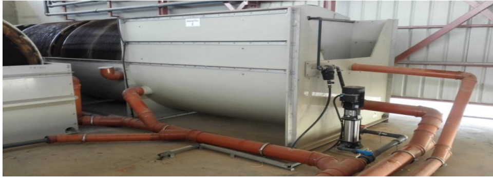
Figure 13: Rotating filter at TRWWTP.
