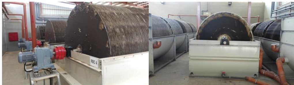
Figure 12 : (RBC) Units at TRWWTP.
