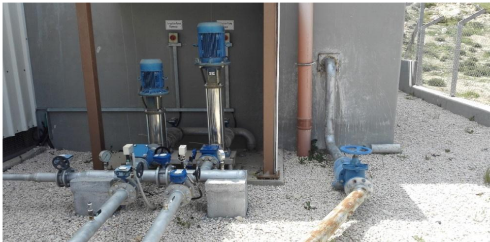
Figure 16: Reclaimed water pumps for Reuse in TRWWTP.
