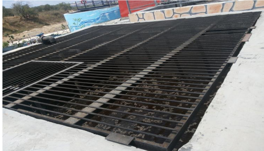
Figure 6: Sludge holding tank in AWWTP
