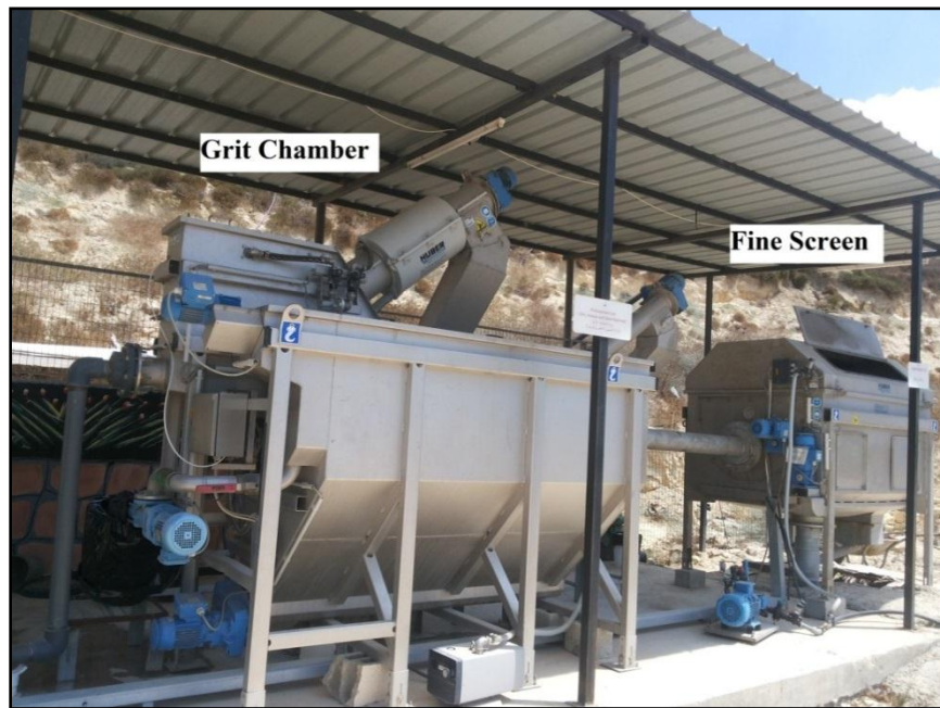
Figure 3: Complete pretreatment unit in AWWTP.
