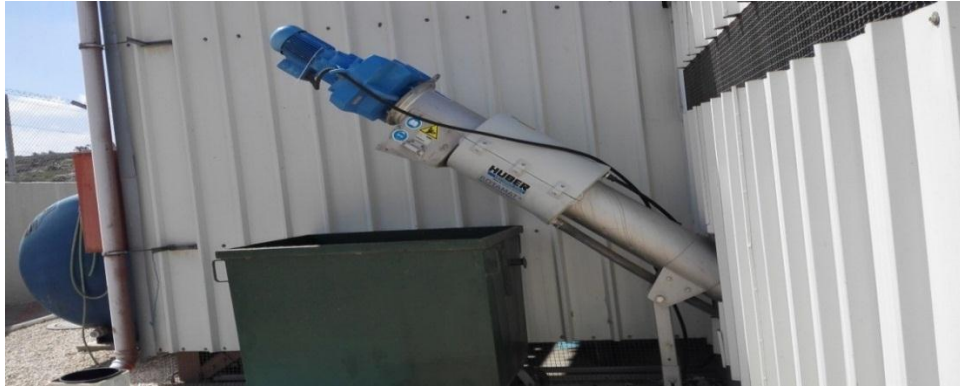
Figure 11: Screening unit at TRWWTP.
